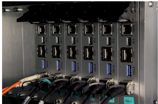
Figure 9b: StarVX parallel VPX computer engine, rear view
